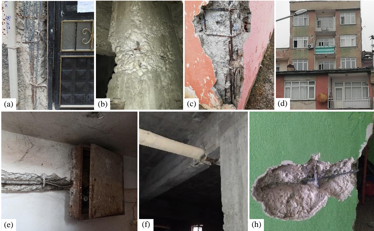
Figure 14: Observed defect examples such as (a) disturbing the column reinforcement due to the door mounting, (b) poor concrete placing, (c) lack of stirrup at the column longitudinal bar extension in the foundation, (d) damage due to the pounding effect, (e) damaging the beam to install electrical cable, (f) damaging the beam to install water pipe, (g) placing the longitudinal rebar out of the stirrup.
