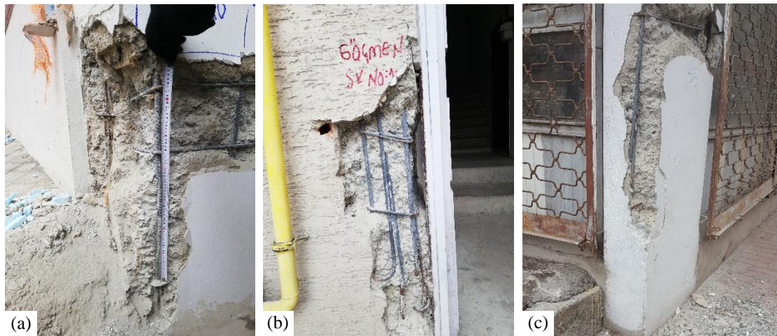
Figure 12: Lap splice defects in damaged buildings in Elazığ; (a) excessive distance between stirrups/stirrup legs, (b) inadequate development length and confinement defects: large spacing and hook angle, (c) 75 cm stirrup spacing at a lap splice.
