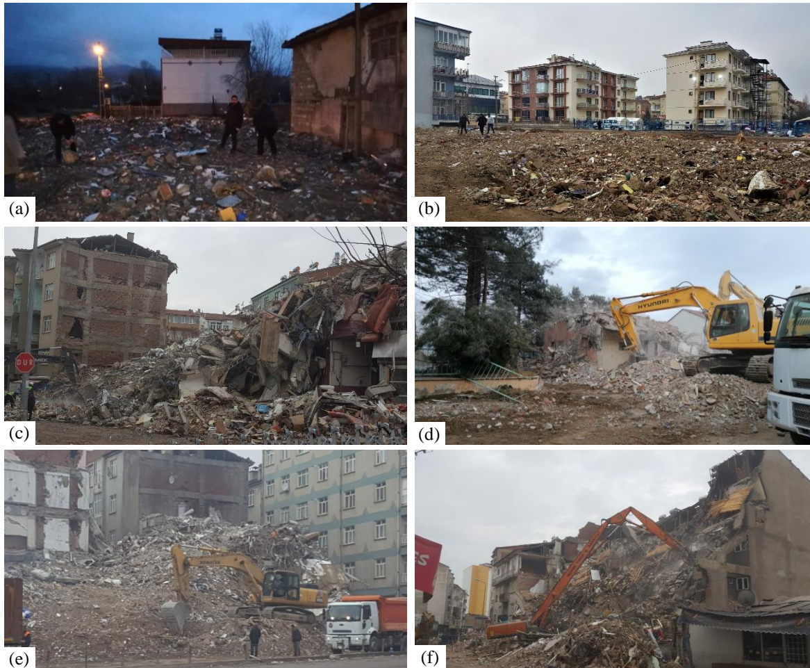
Figure 3: Some of the collapsed and severely damaged buildings from which the material samples were taken in Elazığ; (a) C01, (b) C02, (c) C04, (d) D05, (e) D12, (f) D18.
